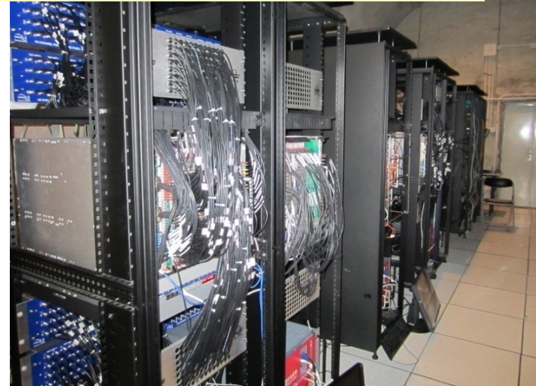
Electronics room in Hall 1
